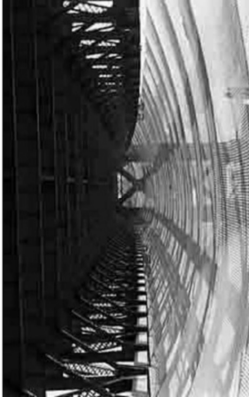
Golden Gate Bridge construction safety net, which ended up saving the lives of 19 workers. (1936)
